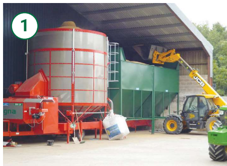
1 A 29 ton automatic dryer with a matched 29 ton wet grain hopper is loaded with wet grain being stored inside the shed behind.
