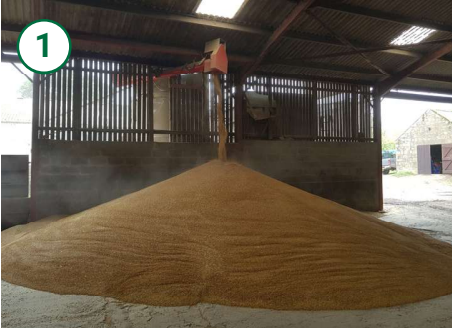
1 A common and low cost system is to discharge from outside a grain store through the cladding above the grain walling.
